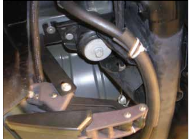
Heater hose for fuel line protection.
