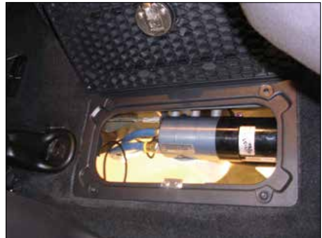
From above, a picture of the FASS unit that I installed on the outside of the driver's side frame rail.
